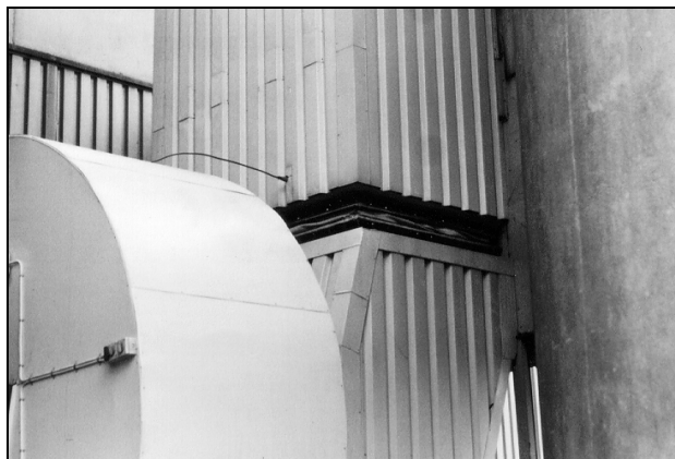
B A. Incinerator Plant. Denmark. Flue Gas Fan. Outlet
