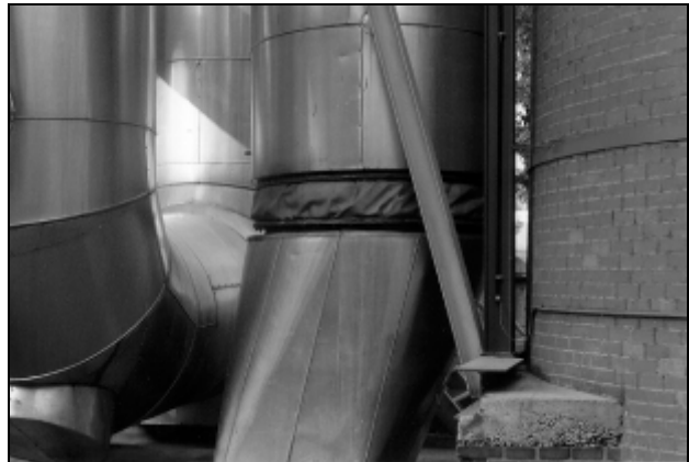
B D. Incinerator Plant. Denmark. Exp. Joints for DeNox System
