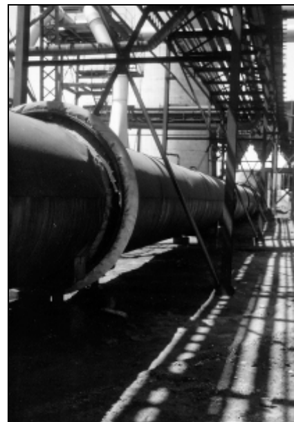
B B. Copper Mine. Botswana. Gas Cleaning. Main Duct. Type IV
